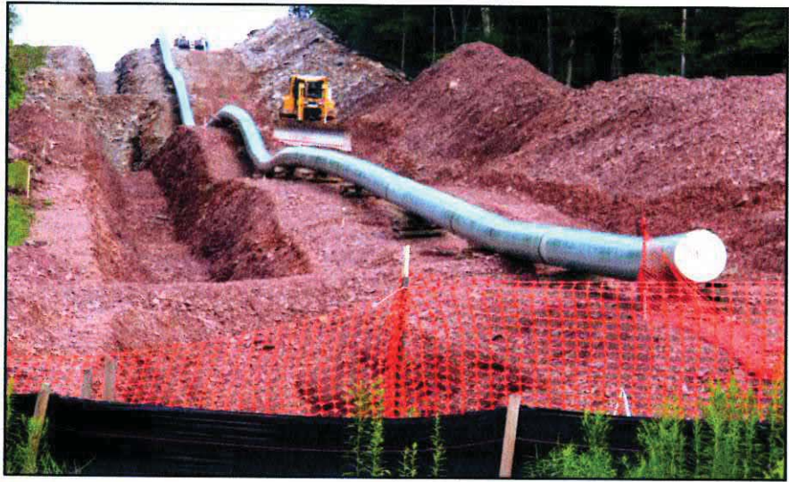
LAYING PIPE: The Tennessee Gas Pipeline Co. was laboring in Wayne and Pike Counties all summer installing new parallel line and pressure stations as part of its 300 Line Expansion Project to transport natural gas through northeastern Pennsylvania. This pipe section above was being prepared at a site off Rt. 652 between Beach Lake and Honesdale in early August. (UDC Photo by David B. Soete)
